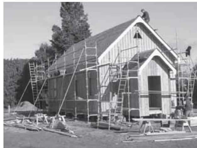
Guided by the conservation plan and Lower Northern NZHPT staff, the restoration work is progressing well. Here, the team from Shingle & Shake Roofing is reinstating the timber-shingled roof. This is part of the plan to take the building back to its near original appearance, given that most of the kauri boards had survived. Photo: K Hearle, 29 July 2011.
