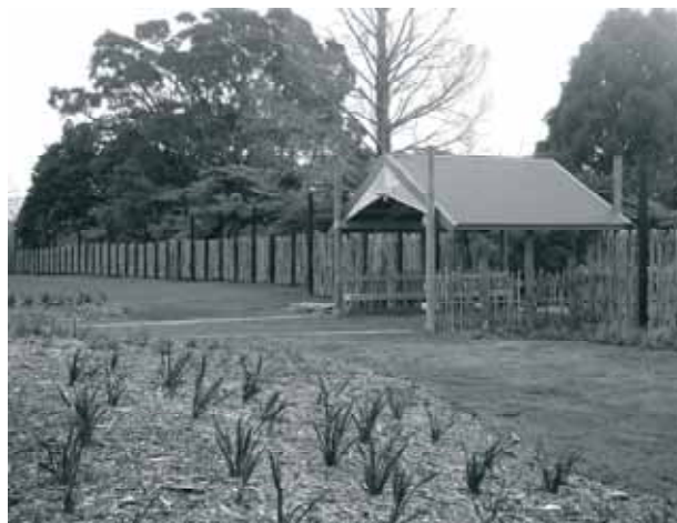
The newly erected waharoa leads visitors across the bridge built to protect the defensive ditch; the palisade type fences were also part of what was achieved in three short days, as were the plantings. Photo: K Hearle, July 2011.
